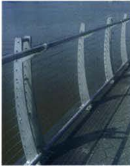
Railing light - Type I railing, illuminated
