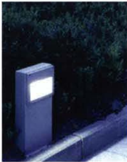
Courtyard lighting - Bollard lights
